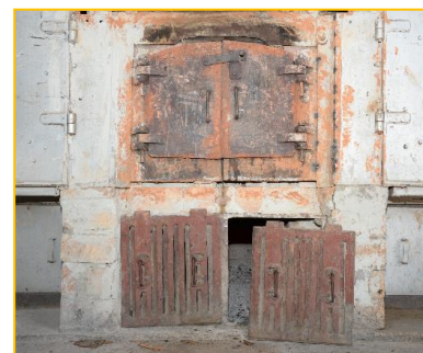
More air leading to energy loss
